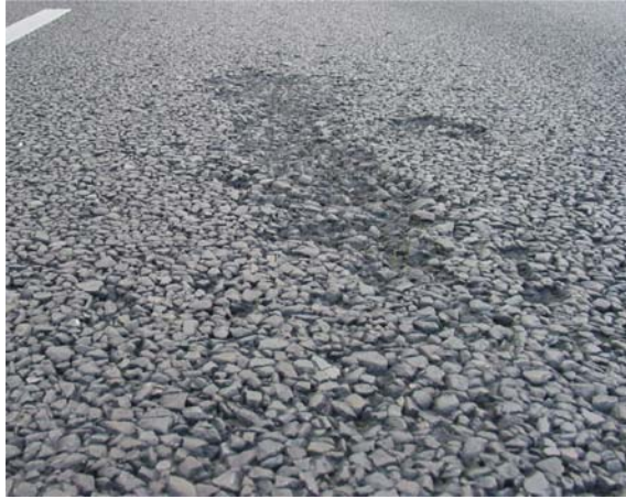
Figure 2: Raveling of the asphaltic wearing surface
