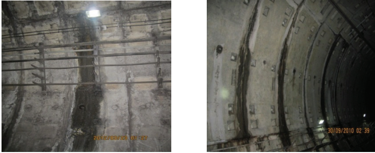
Figure 1: Leakage of shield driven tunnel in Shanghai, China
