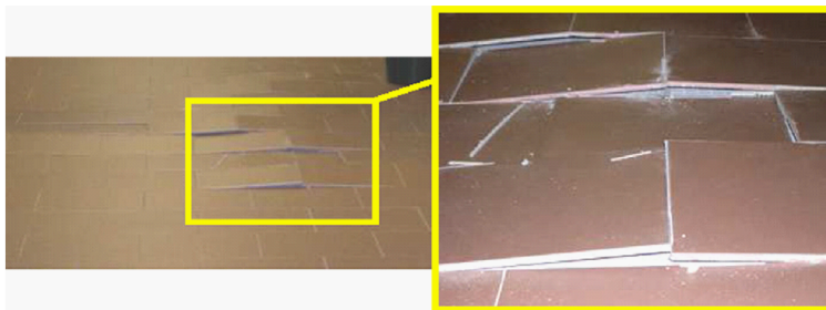
Figure 2: Tile separation from the sub-base in a radiant heat floor [Cocchetti, Comi, and Perego (2011)]
