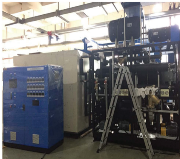
Figure 4: Heat exchanger test bench
