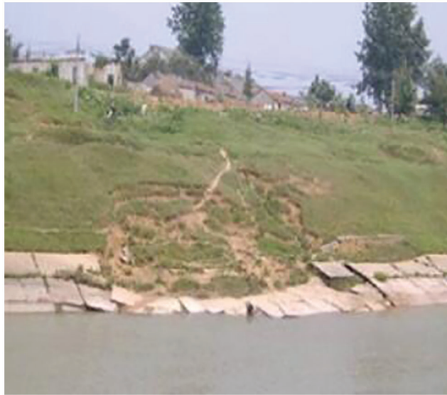
Figure 1: Cutting slope slip
