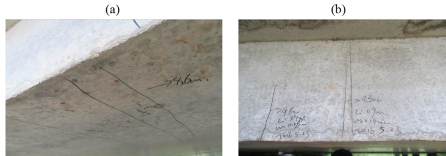
Figure 7: (a) Vertical cracks on web of box girder near mid-span, (b) Vertical cracks on web of the girder #2
