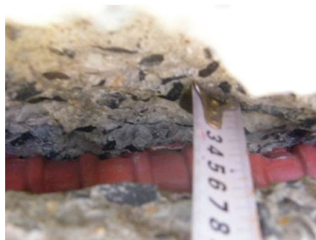
(c) Span No. 2 longitudinal crack corrugate pipe deterioration
