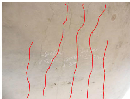
(a) Span No.2 bottom slab cracks ( L=20.5\text{m} \delta=4\text{mm} )
