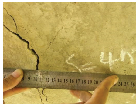
(b) Span No.2 longitudinal bottom crack ( L=0.7\text{m} \delta=0.6\text{mm} )
