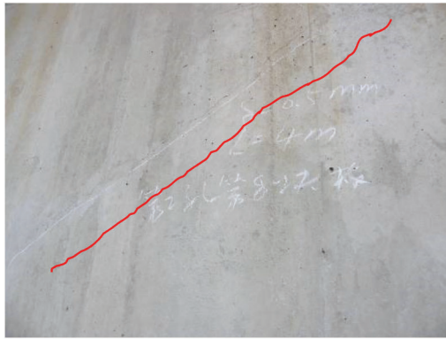
(a) The crack observed on the exterior surface of block No. 8 ( L=4.0\text{m} \delta=0.5\text{mm} \alpha=45^\circ )
