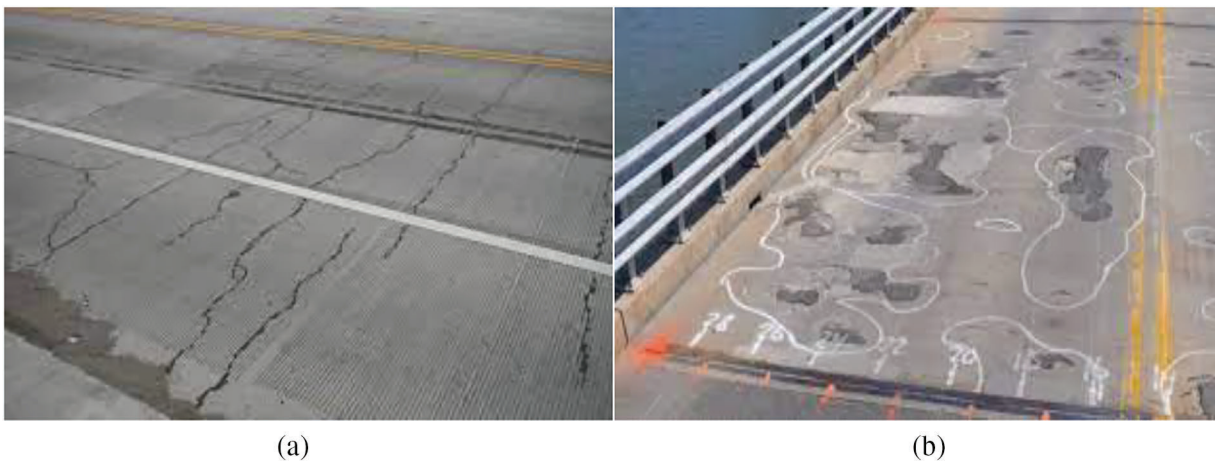
Figure 8: (a) RC deck with cracks, (b) spalling and potential delaminations. Reprinted from Reference [6]
