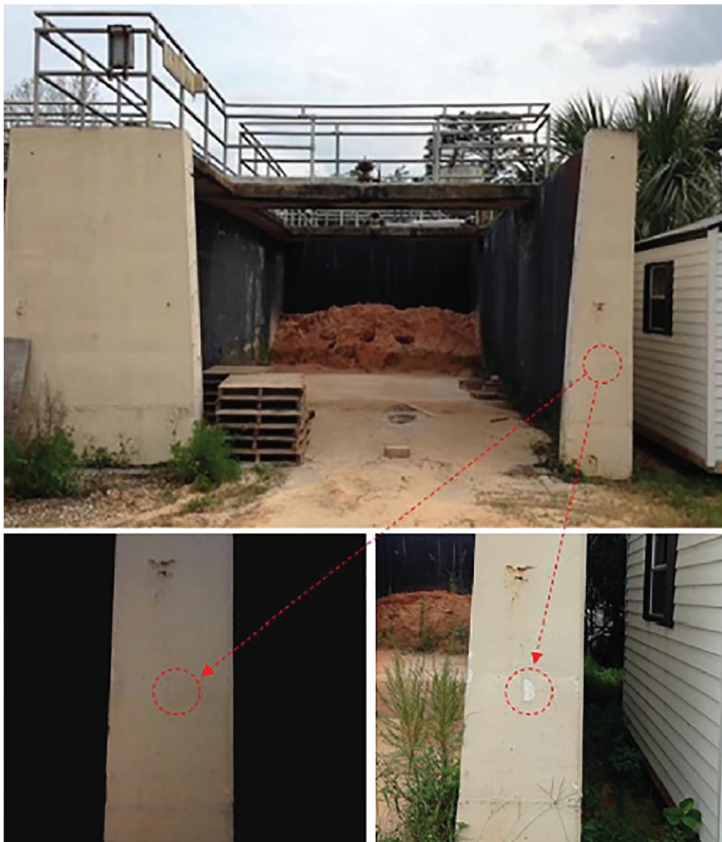
Figure 23: Concrete structure with delaminations. Reprinted from Reference [95]
