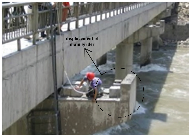
Figure 34: The maximum displacement of bridge in Dujiangyan. Adapted from Reference [48]
