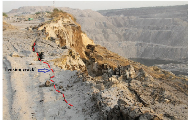
Figure 1: A typical view of tension crack near the pit slope edge of an open cast mine of Godavari valley coalfield, India
