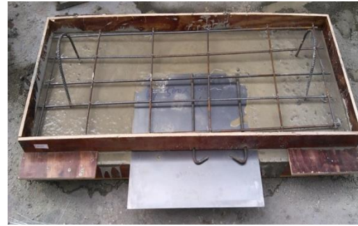
(b): The steel plate with 500×400×3mm dimensions was placed in the middle part of the track plate
