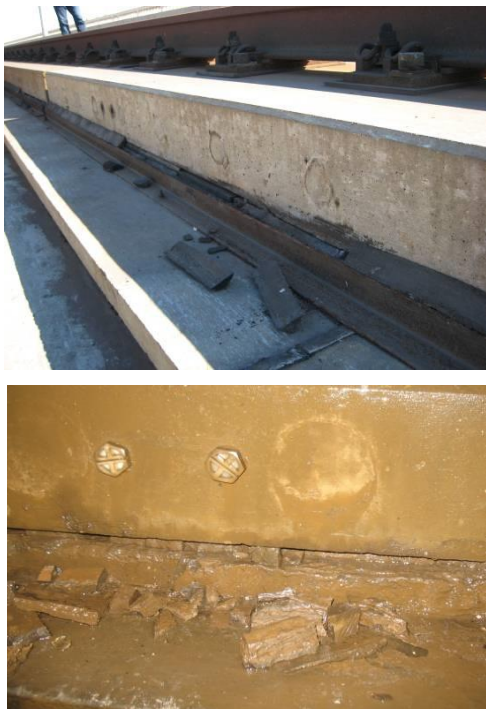
Figure 2: Example of damages on non-ballasted track. Shown is Cheng-yu line. The left panel depicts water accumulation between the supporting layer and the CA mortar, and the right one presents a crack on the track plate
