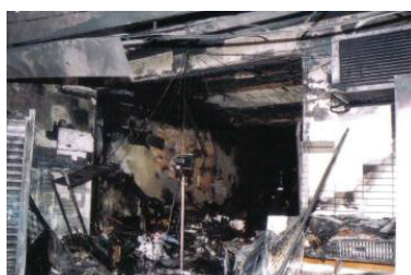
Figure 9: Room 2 after accident burning of the fire
