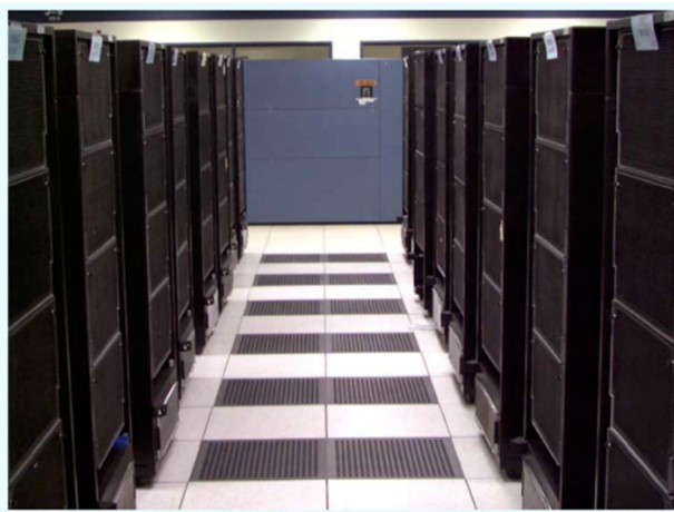
Fig. 1 View of a typical cold aisle in a data center.
