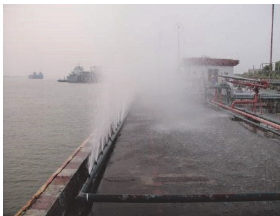
Fig. 1 Photo of water curtain switched on in an oil and gas terminal
